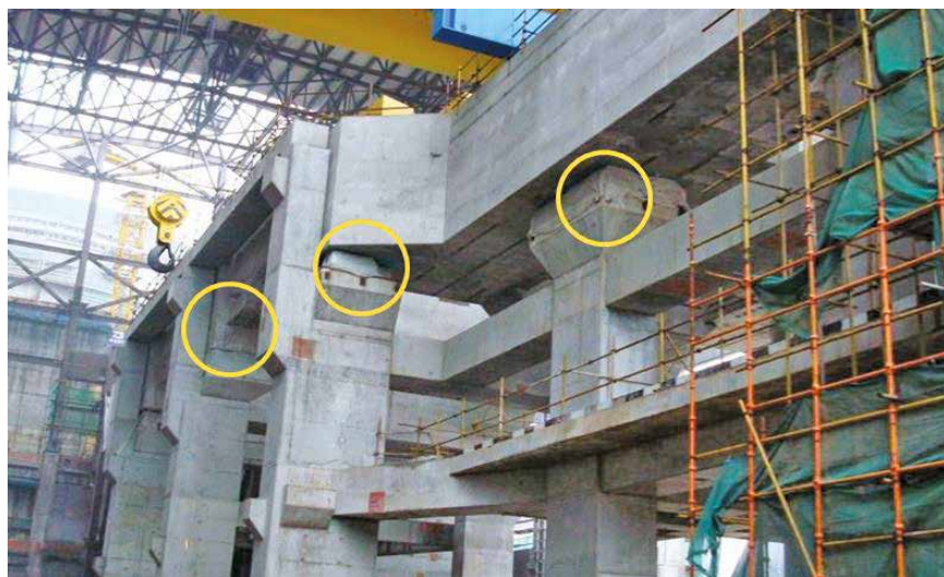
Fig. 10-18. Ling Ao Phase II, 1000 MW turbine tabletop on VIS, China Source: Courtesy of GERB Vibration Control Systems; reproduced with permission.
