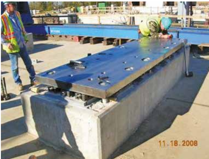
Fig. 11-11. Baseplate/soleplate placed on top of vertical alignment devices Source: Courtesy of Robt. L. Rowan & Assoc., Inc.; reproduced with permission.
