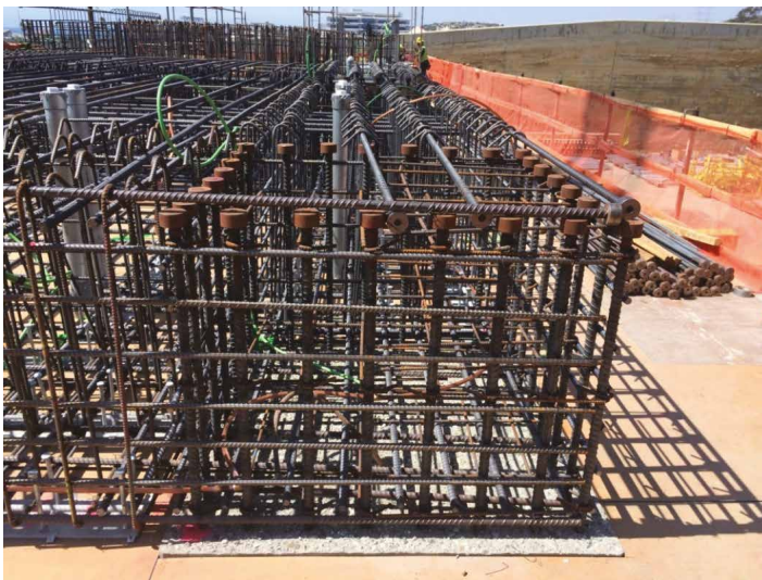
Fig. 11-2. Example where headed reinforcement is used in congested joint Source: Courtesy of Kiewit Engineering Group; reproduced with permission.
