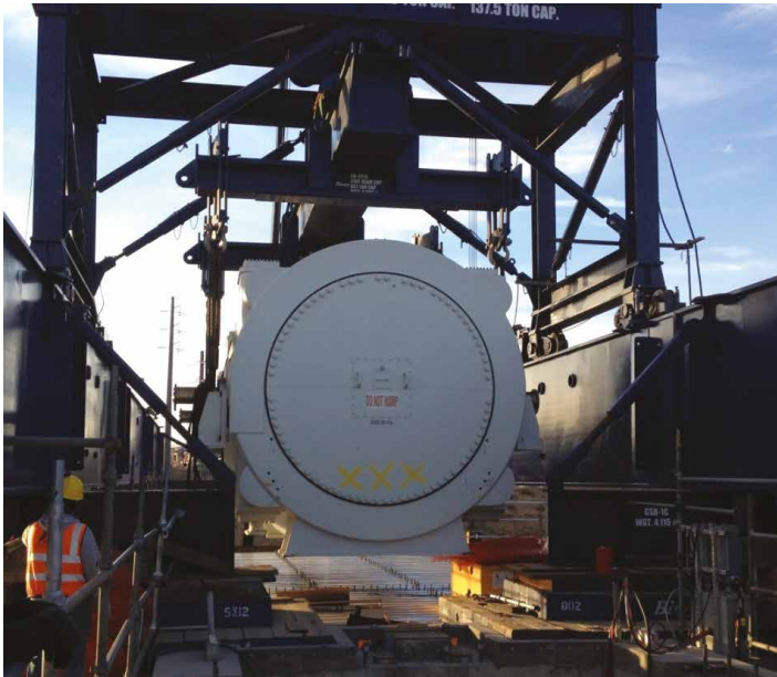
Fig. 11-5. Generator installation with gantry system supported off tabletop Source: Courtesy of Kiewit Engineering Group; reproduced with permission.
