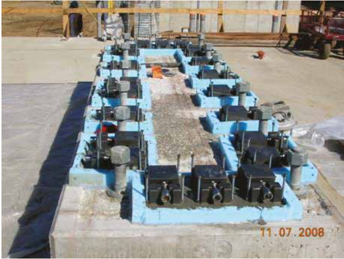
Fig. 11-10. Vertical alignment devices set up and grouted into place Source: Courtesy of Robt. L. Rowan & Assoc., Inc.; reproduced with permission.
