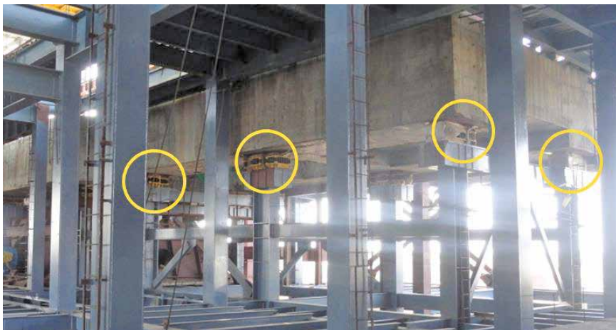
Fig. 10-17. 660 MW turbine tabletop on VIS integrated into machine building, Jhabua, India
